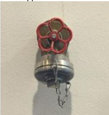
Dry riser (inside)
