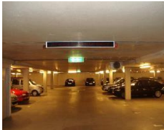
Warning light with flashlights in the underground car park
